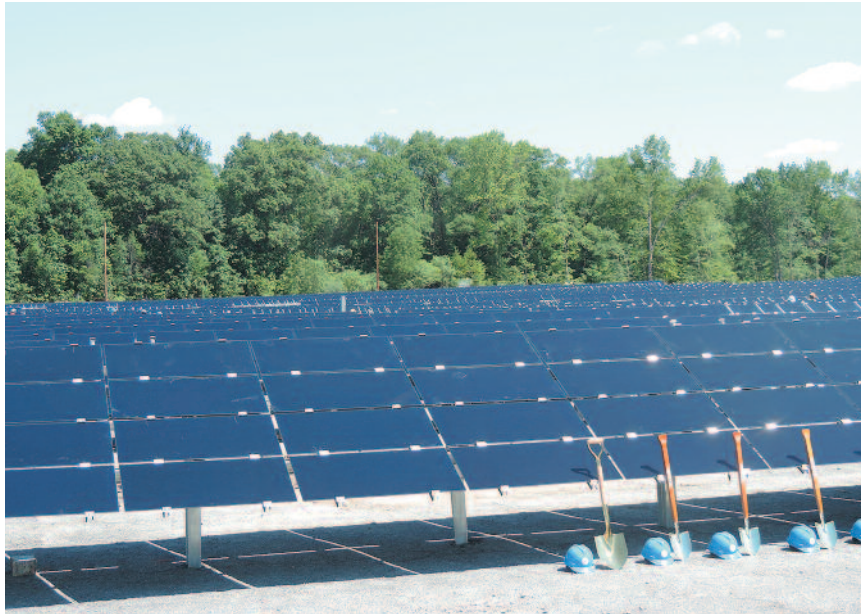
A total of 19,020 solar panels will enable President Container Group to save 25 percent annually on the electricity required to power its 522,000-square-foot super plant.
