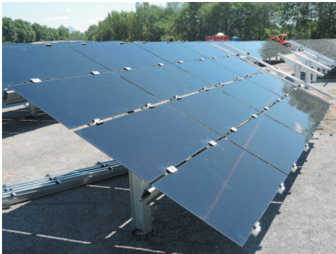
One of 951 'tables,' each holding 20 2-foot by 4-foot solar panels.
